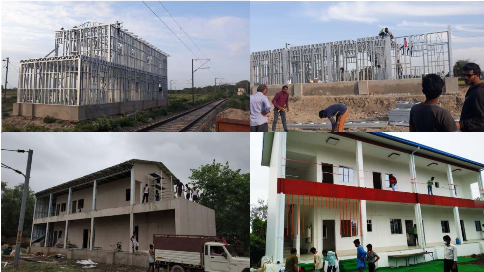
Railway Office & Signaling Room
